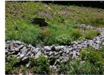
Remove sediment build-up at inlet headwall forebay. Clean/turn rip rap at inlet headwall forebay.
