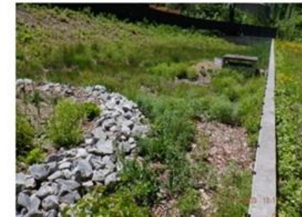
Remove sediment build-up throughout pond to ensure water flow is directed towards OCS.
