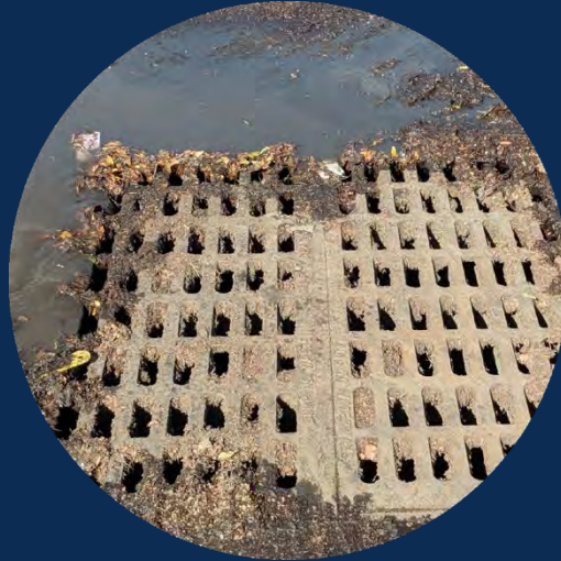
Aging & Undersized Infrastructure
